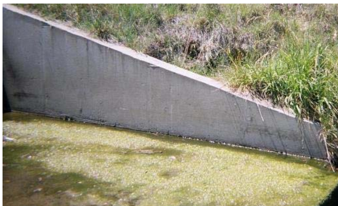
A blanket of Blanket Weed on the outlet of a Gross Pollution Trap.
